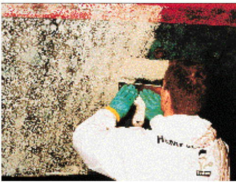
The preparation of the surface to paint is essential to achieve good results.
