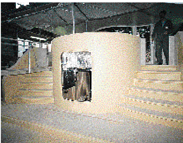
Several coats of epoxy profiling primers are needed for a good finish.
